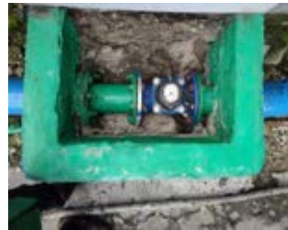
SFB Paddle Cold Water Meter (Pump 3)
